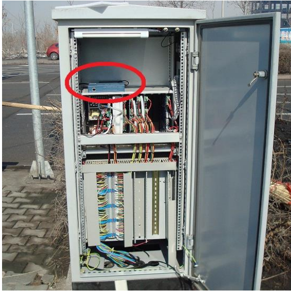
Installed inside the signal controller for signal control.
