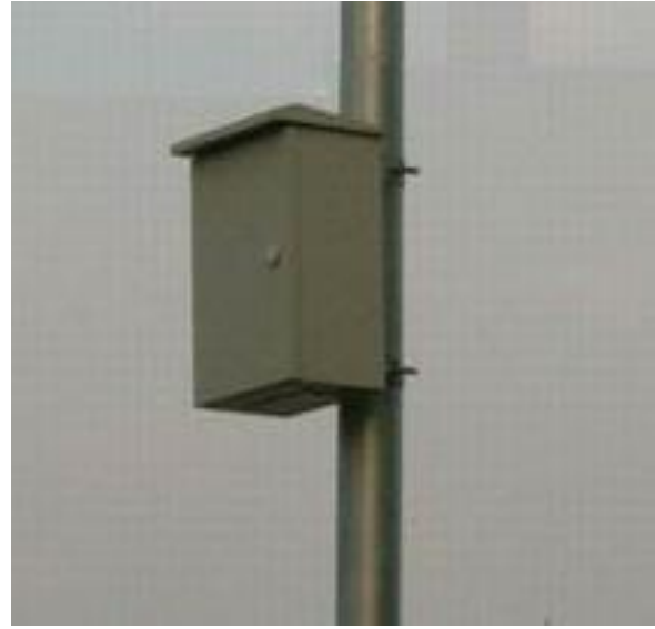
Installed inside the cabinet for road segment traffic flow detection.
